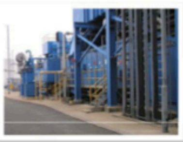
Gas Turbine Package
