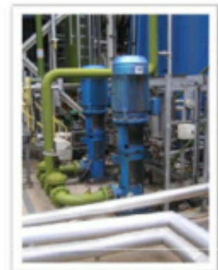
Condensate Extraction Pumps
