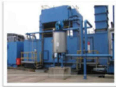
Gas Turbine Generator
