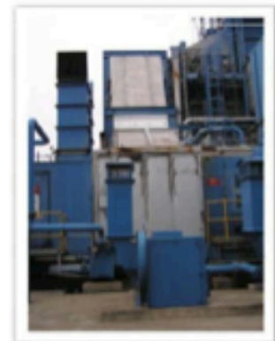
Gas Turbine Exhaust
